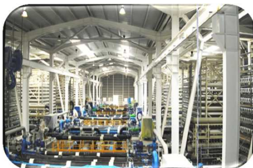
200,000 m 3 /day desalination plant. (Honnaine, Algeria)
